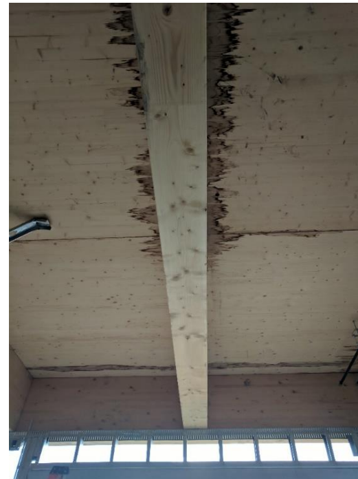
Photo 7: Staining at panel edges from exposed joint above.
