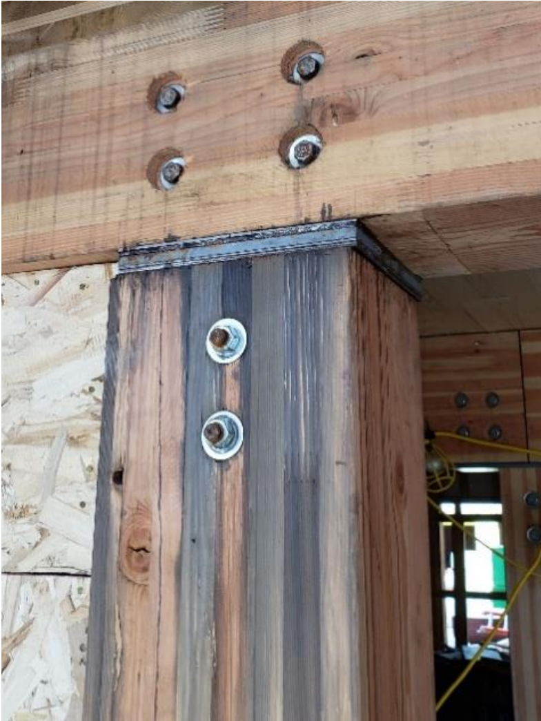
Photo 2: Staining from corrosion of metal connectors.
