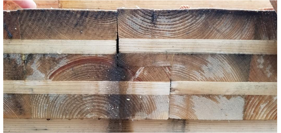
Photo 3: End grain staining from an exposed CLT joint.
