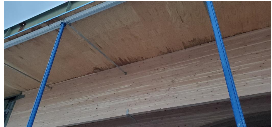
Photo 5: Staining on exposed underside of CLT from end grain absorption.
