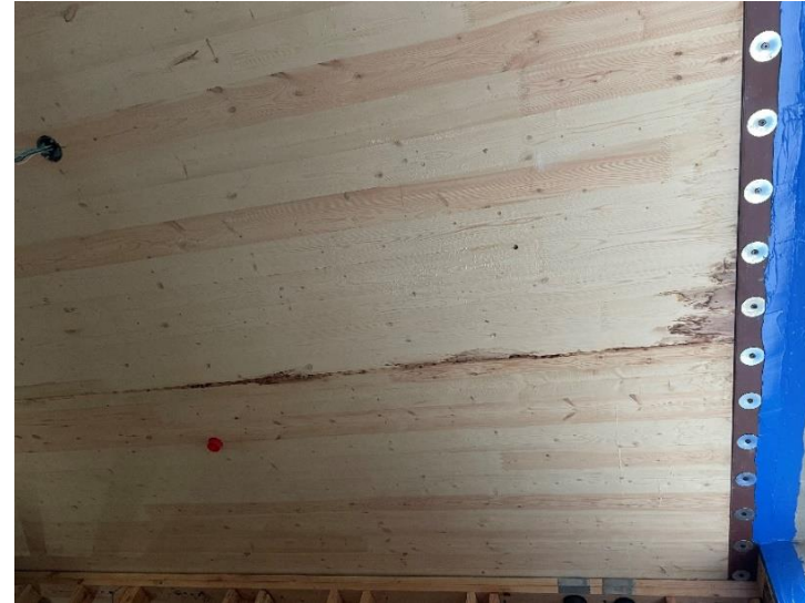
Photo 6: Staining at end grain and panel joints with side grain.
